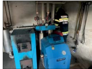
Heizraumbrand in Kocheregg
